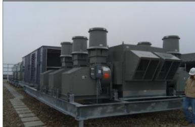
Custom MUA unit with heat recovery/lab exhaust
